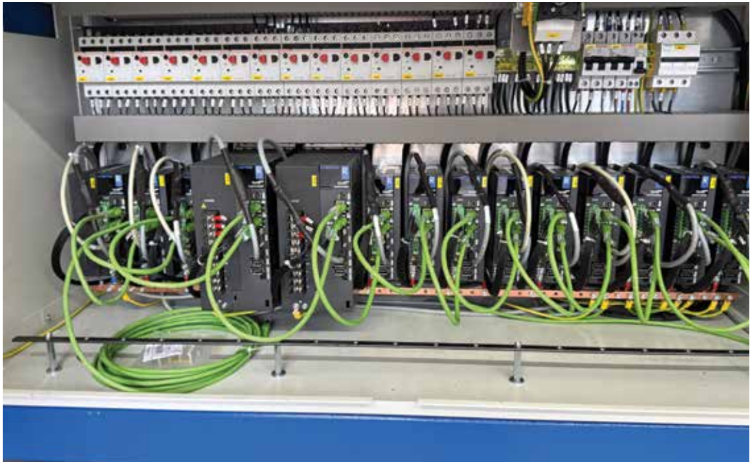
Digital drive controllers
