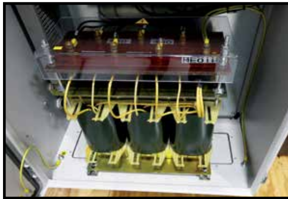
Incoming power transformer
