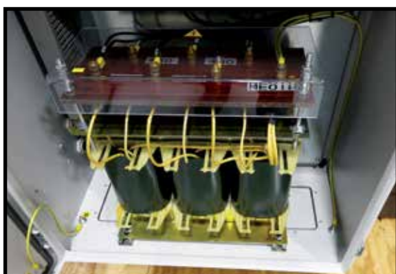
Incoming power transformer
